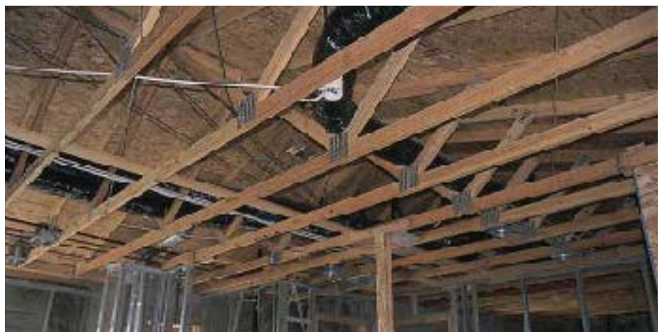
Figure 4. While bearing walls and partitions are framed with steel, I-joint floors (top) and conventional wood roof trusses (bottom) save money on fasteners and permit an efficient framing sequence.
