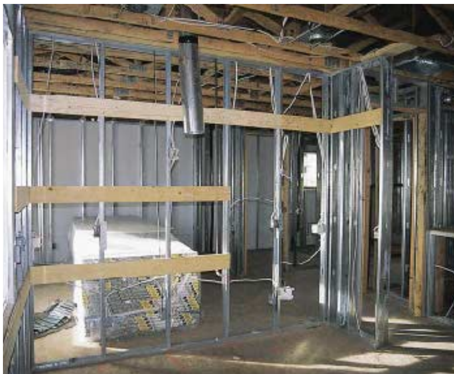
Figure 10. Plywood strapping, screwed to the studs before the drywall goes up, provides a solid base for kitchen cabinets.
