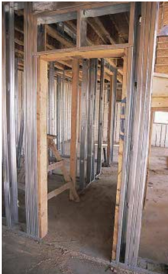
Figure 9. To provide solid nailing for door trim, openings are blocked with 2x4 material on three sides.
