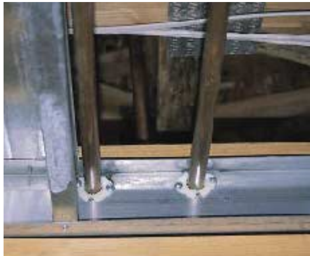
Figure 6. Plastic grommets also isolate the copper water lines from the steel framing (left). A plasma cutter is the tool of choice for making large-diameter openings for drain lines (below, left).
