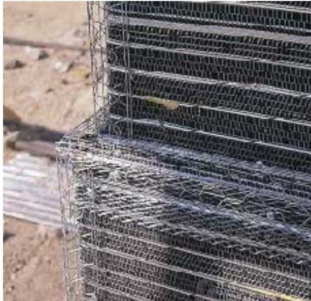
Figure 7. Screws secure the stucco lath to the steel frame. An underlying layer of 7/16 inch foam board provides a thermal break between the conductive steel studs and the exterior finish.
