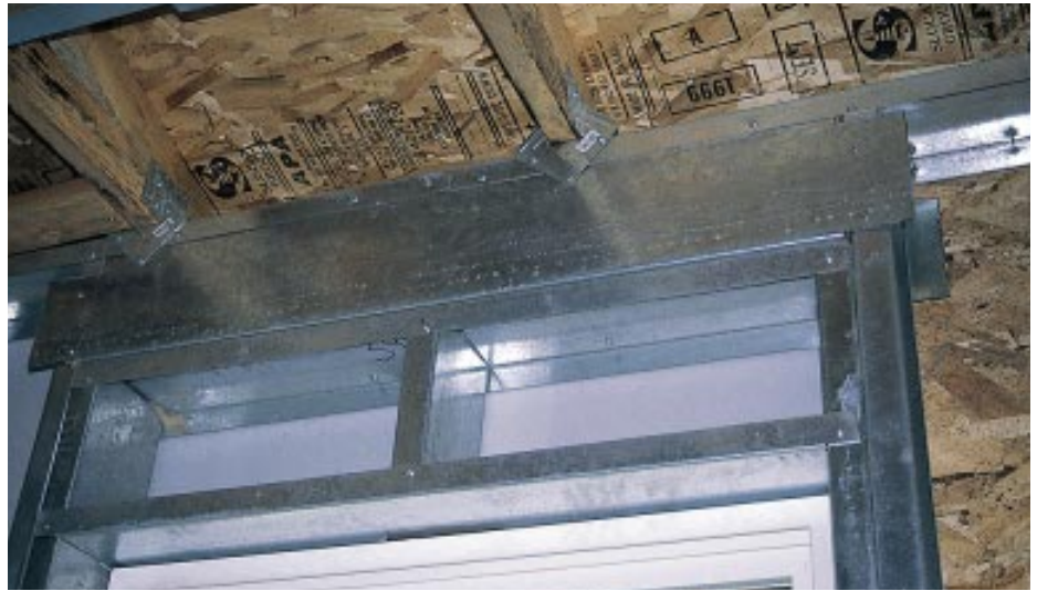
Figure 3. Cripples extend downward from the header beneath the top plate, and terminate at the rough opening.
